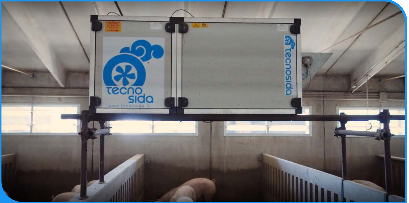
Figure 5. Dry filter system that was installed in the Italian pig farm
