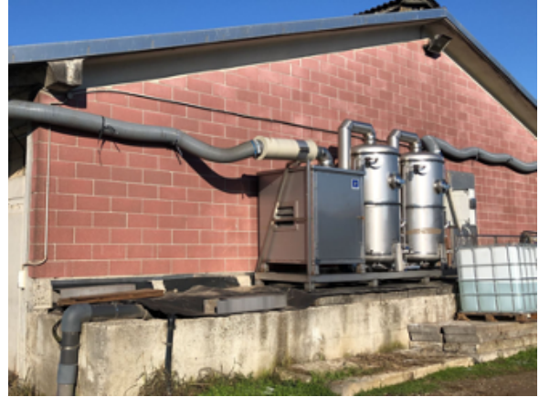
Fig. 4 Wet scrubber installation in Italy
