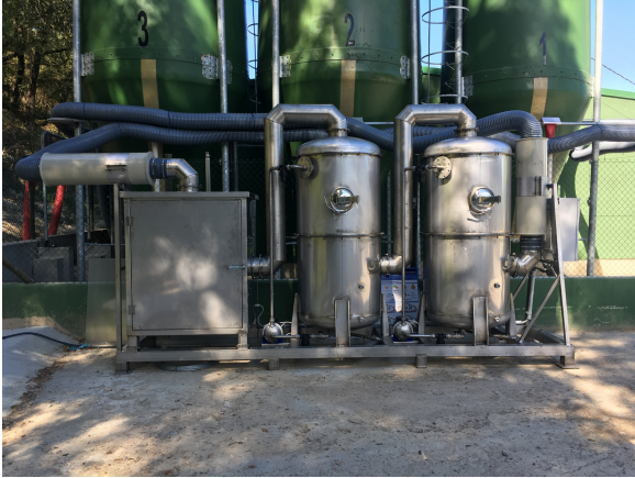
Fig. 1 Wet scrubber installation in Spain
