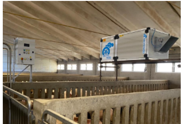
Fig. 5 Wet scrubber installation in Italy
