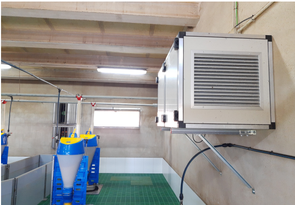
Fig. 2 Dry scrubber installation in Spain
